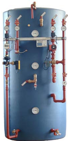
District heating station
