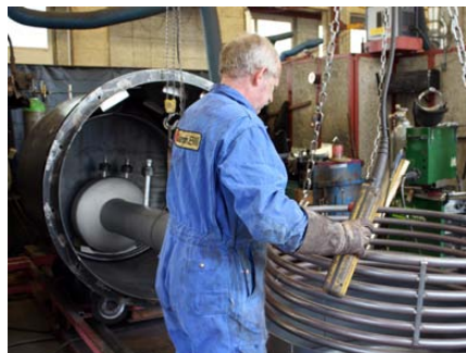
Heat exchanger, boiler and connections are welded
