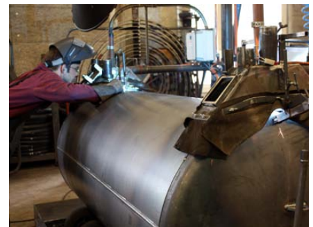
In the case of a tank without internals, lids and bases are welded at the same time
